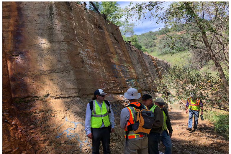
Concrete dam on Chaparral Gulch holding back a wall of tailings in the flood plain above.
