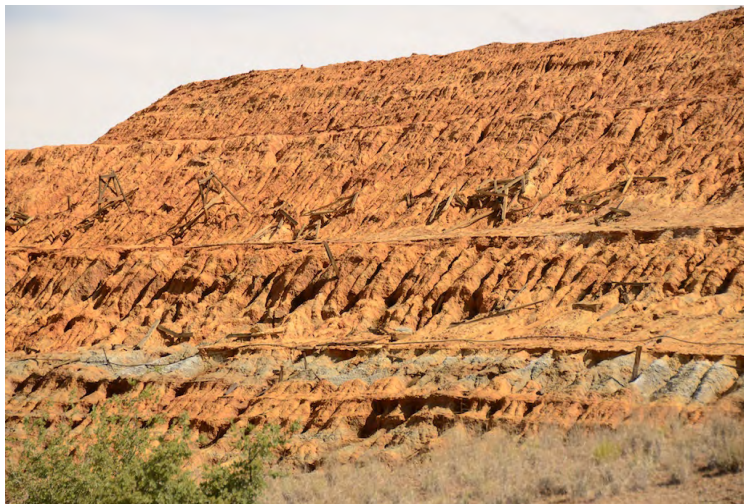
Side of Iron King Mine tailings pile as seen from the north.
