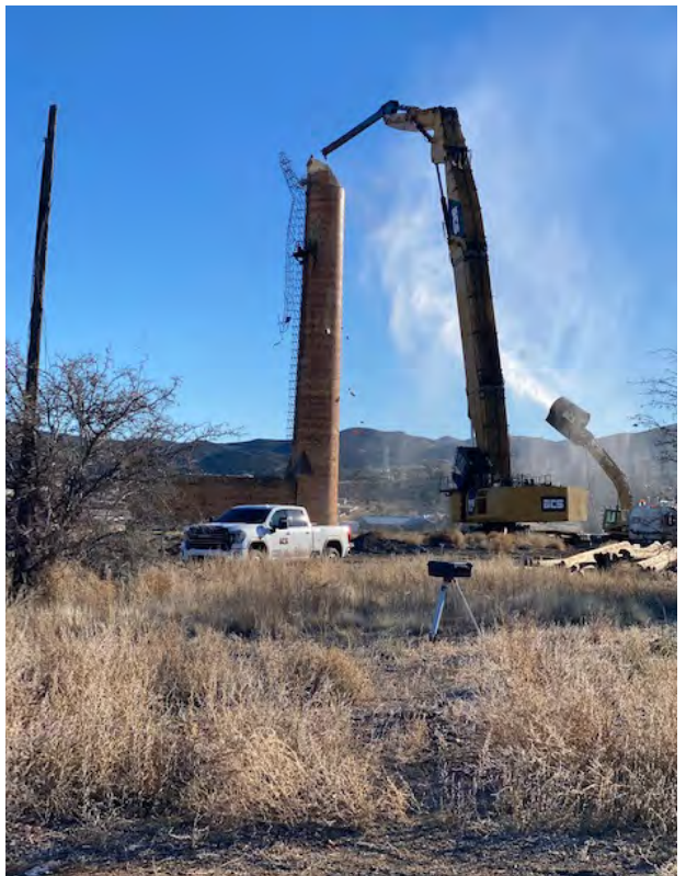
The ADEQ dismantled the remaining Humboldt smelter stack in 2022 as it was unsafe and attracting people to a contaminated area.
