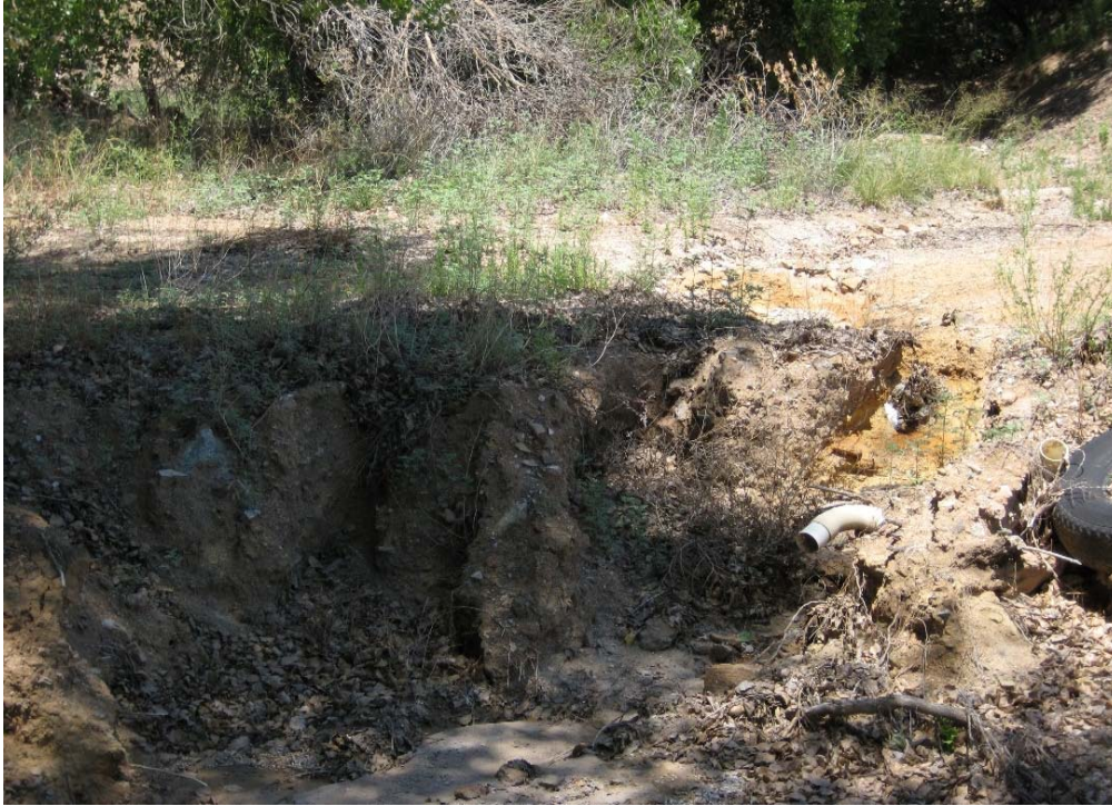
Photograph 9: Unnamed drainage near Blowout Path at VP8
