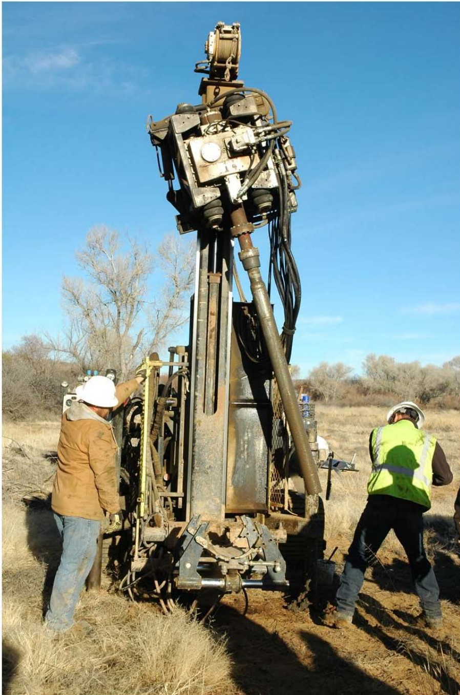
Photo DSC_0643: Photos during investigation: depicting percussive drill rig used to obtain cores from the ground in the Iron King Mine Blow Out Path
