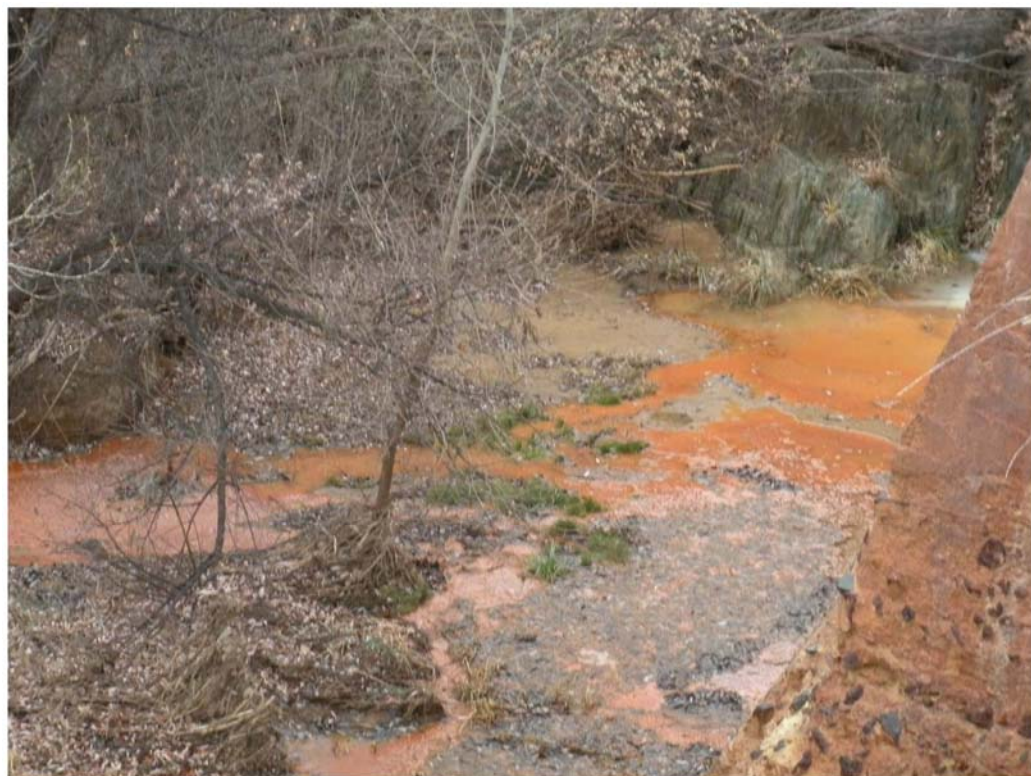
Photo F004: Ponds of water at the base (downstream) of Chaparral Gulch Dam
